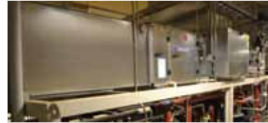
Air conditioning units
